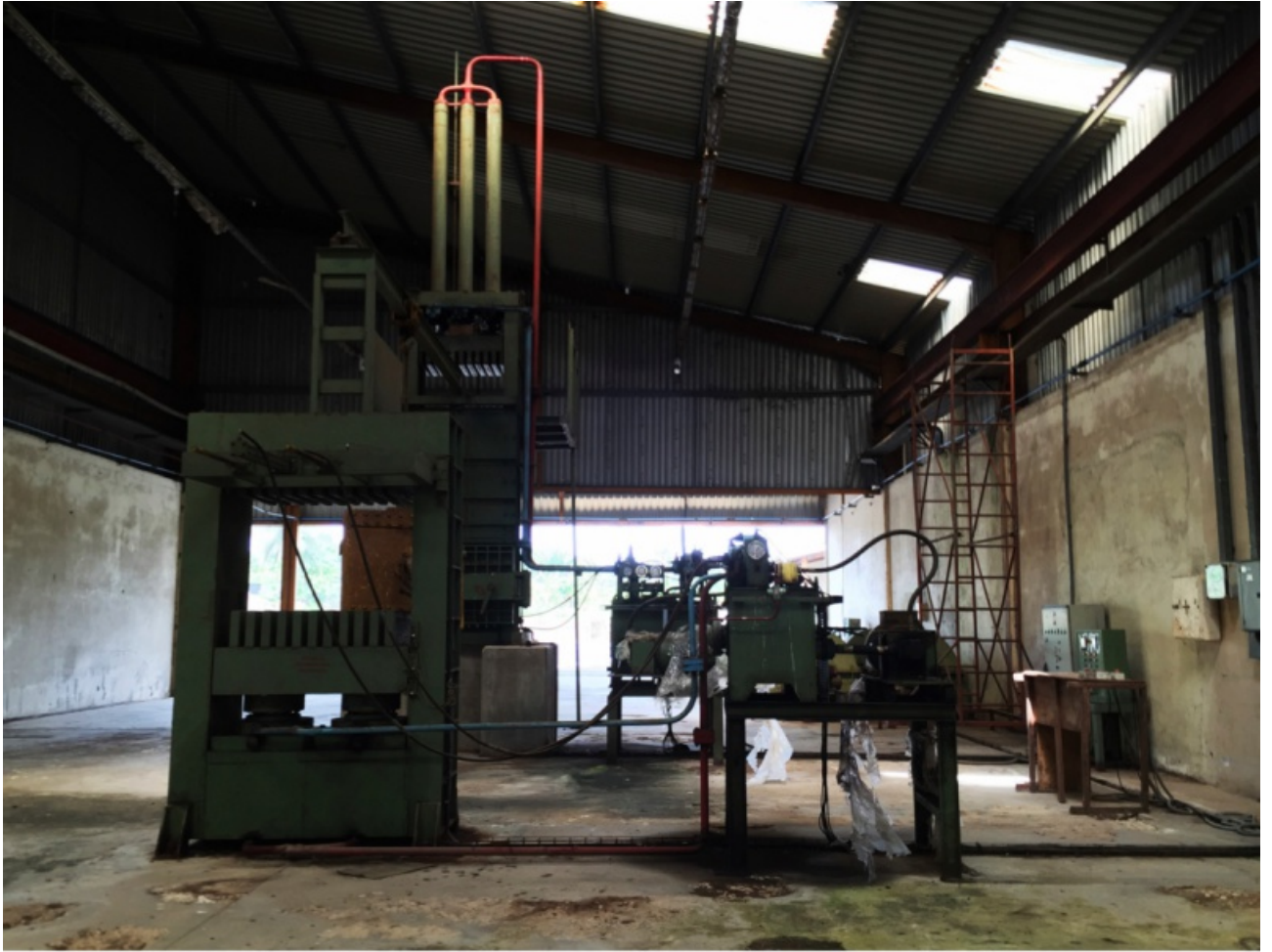
Coconut Husk Production Equipment in Decommissioned Factory Tikobo 2, Ghana, 2014 Photo Credit: Mae-ling Lokko
